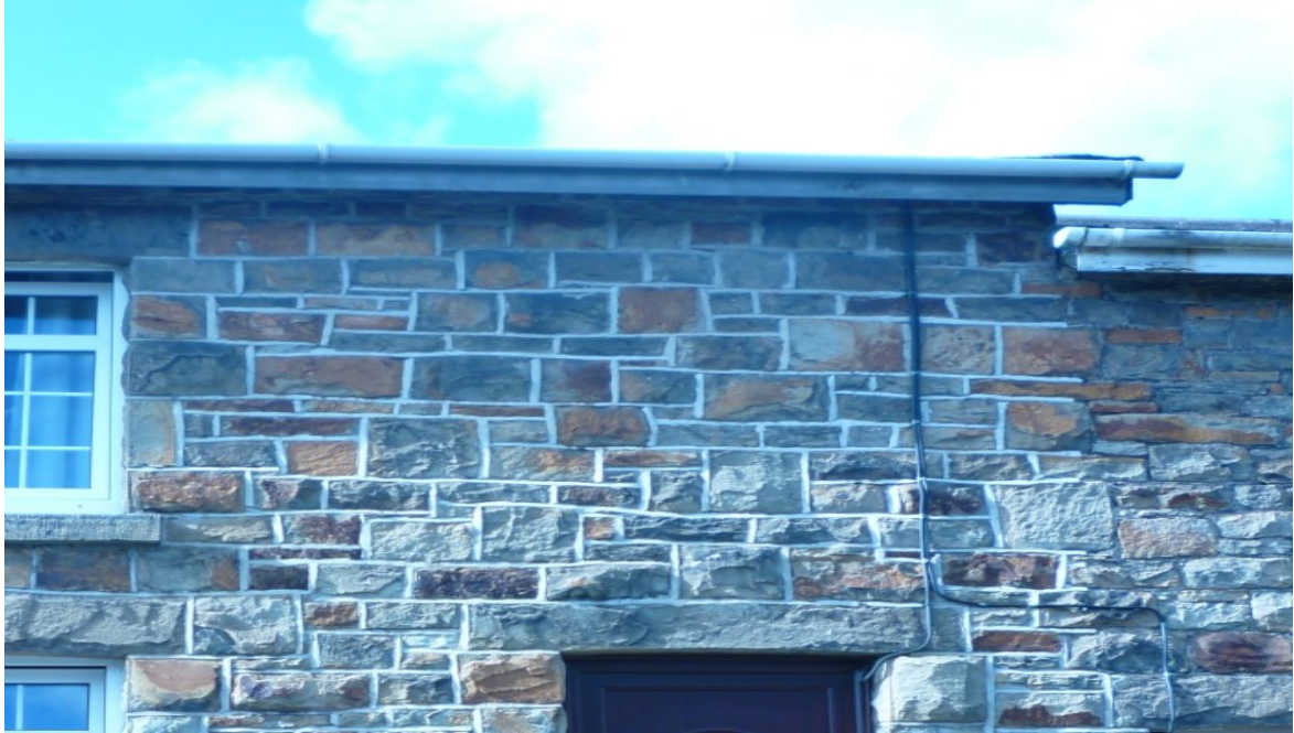
Fig1.14: Pointing surface in wall
